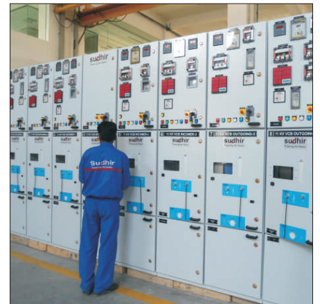
33 kV HT Panel
